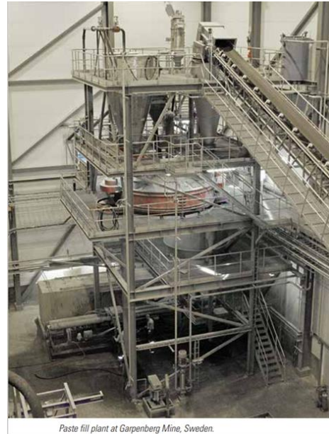
Paste fill plant at Garpenberg Mine, Sweden.
